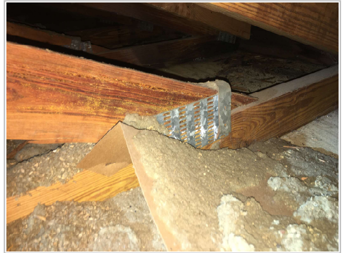
Toe Nail - Not Meeting Nail Requirements
