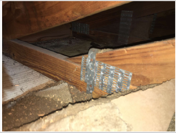
Toe Nail - Not Meeting Nail Requirements
